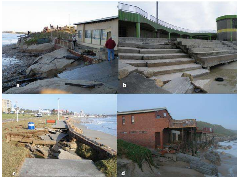
Figure 6 Threat to infrastructure placed too close to the sea through erosion at a) Summerstrand lifesavers clubhouse, b) New Brighton Beach facilities and wave attack at c) seawall and walkway east of hobie beach and d) clubhouse facilities at Sardinia Bay.
